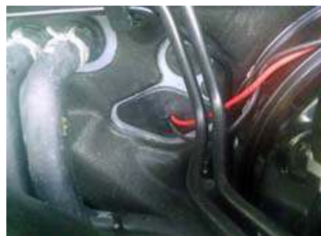
Power cables pass through the firewall grommet on their way from Yaesu radio to vehicle battery. [Pic - N2CBH]
