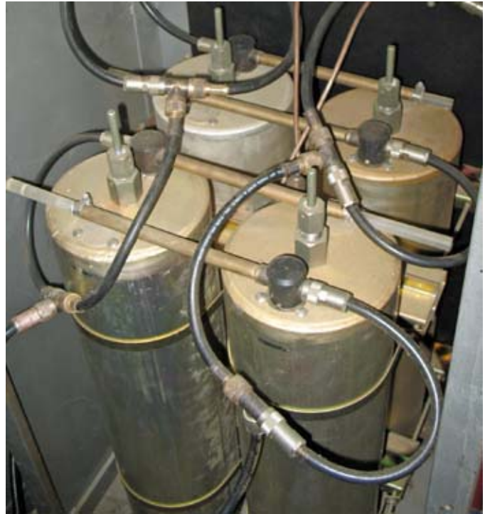
Part of the six-cavity duplexer currently in use on the 2 meter test repeater. Bob N2CBH was able to tune this set of cavities to 146.67/146.07 MHz.
