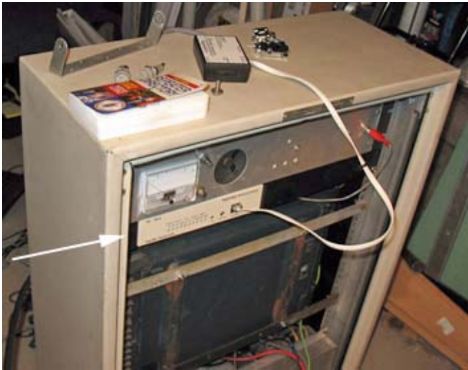
Pacific Research Solutions repeater controller in the 2 meter test machine is shown arrowed.
