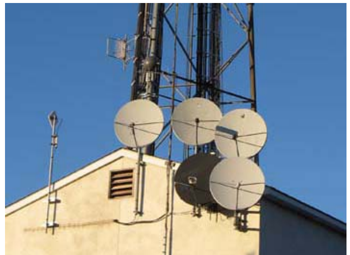
Antennas in the sunset. A view of the N2CBH/R and W2NYW test repeater location.
