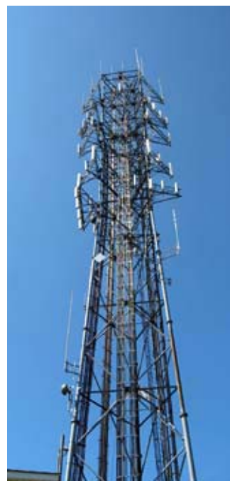
Tower at the new site. Antenna is at lower left.
