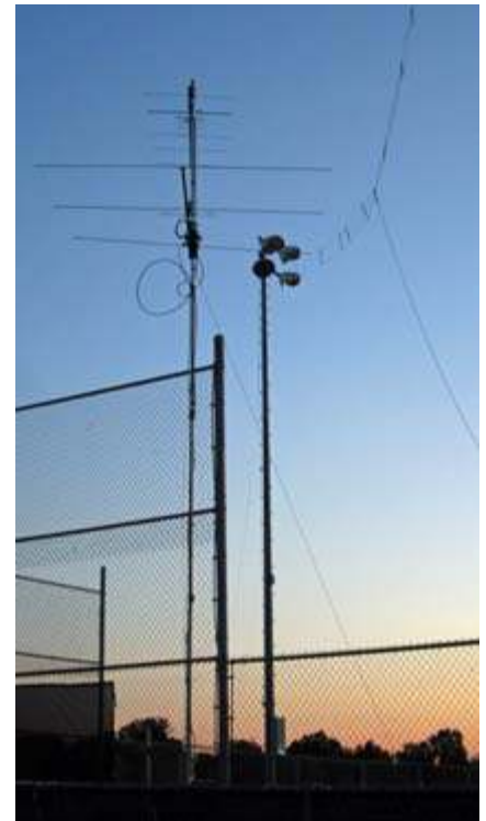
Evening view of the VHF antennas and nearby multi-band dipole.
