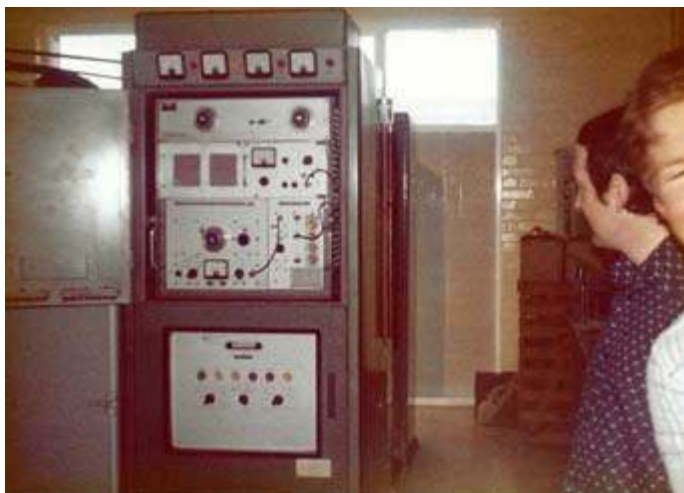
One of the transmitter racks at Anglesey Radio. Just visible on the right, Brian G3SZV and David (then) G8HUP.
