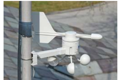
Wind sensor was fastened to an existing 1¼" mast high on the roof.
