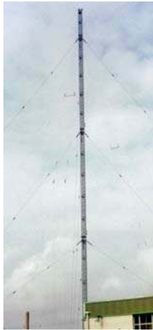
MF transmitter mast at Moorside Edge, England has steel guys broken up with multiple insulators.
