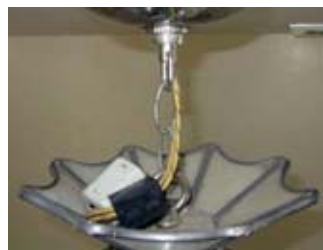
Ferrite chokes clamped over ceiling lamp cable.
